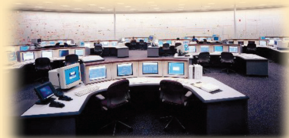
Utility Control Room
